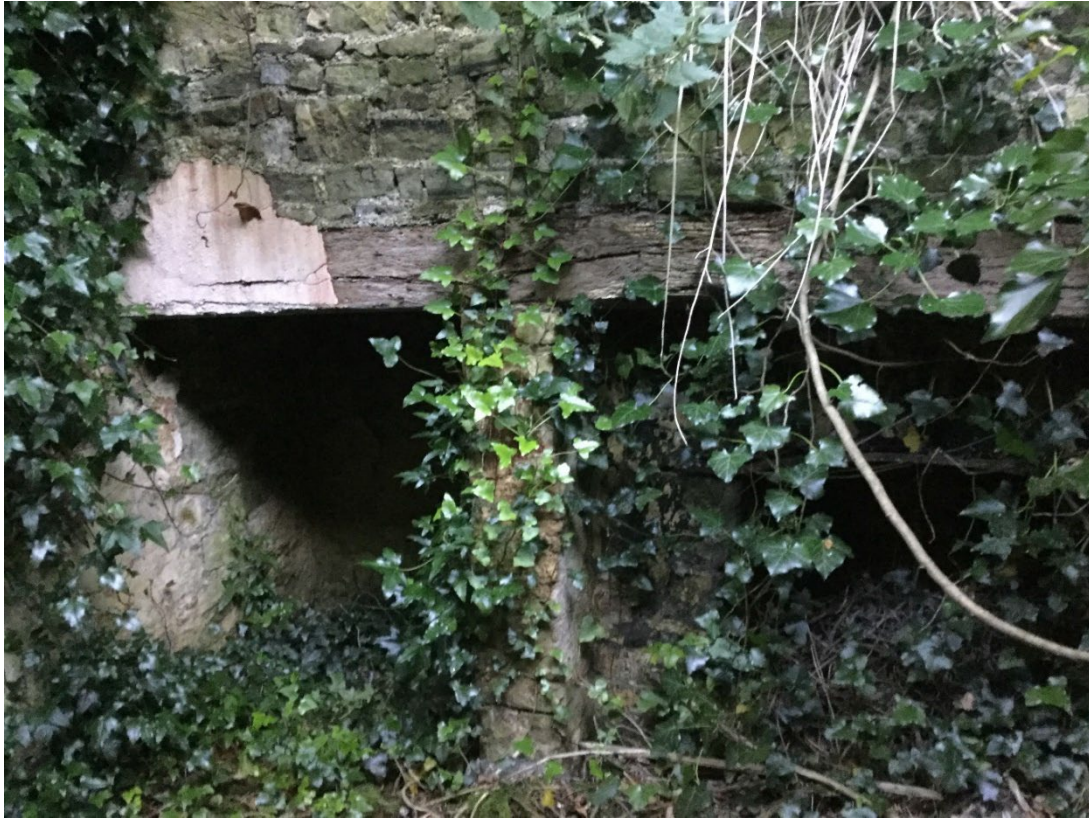
Plate 7. View of the area beside (left) the fireplace with a high roof which is enclosed in Building B
